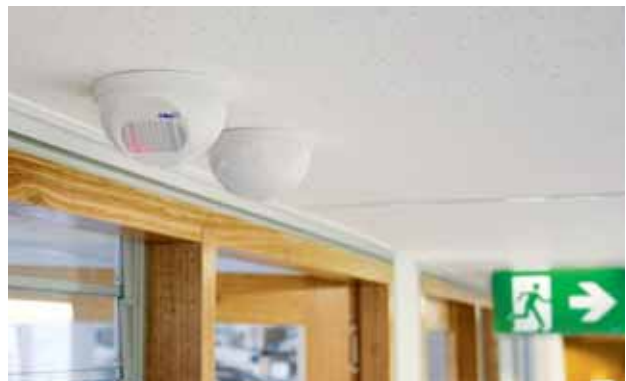
Only as needed: timers, movement and photo-electric light sensors ensure efficient use of lights in the common areas.
